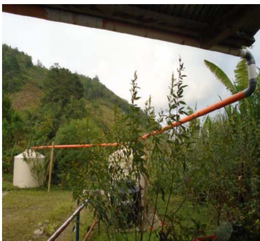
Rainwater harvesting system
